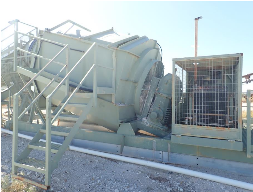
Figure 1: Agitator machinery with guarding on engine and driveline components
